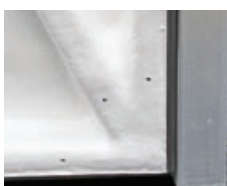
The "flowcoat" provides a smoother finish as shown on the bottom corner detail illustrated left
